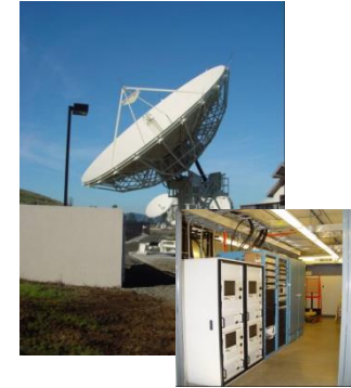
4 Ground Earth Stations
